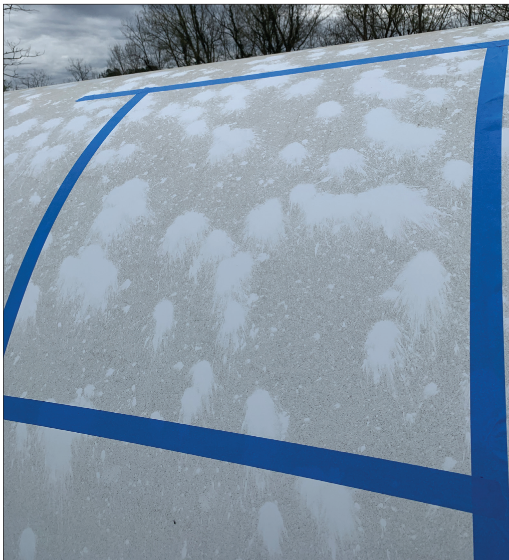
Figure 1. Image displaying hail-strike markings on the storm shelter located in Camp Hill, AL, ~2.6 km from the Auburn Captive Facility. Blue tape represents boundaries of 1-m 2 box used for hail counts. Photograph © Matthew T. McDonough.
